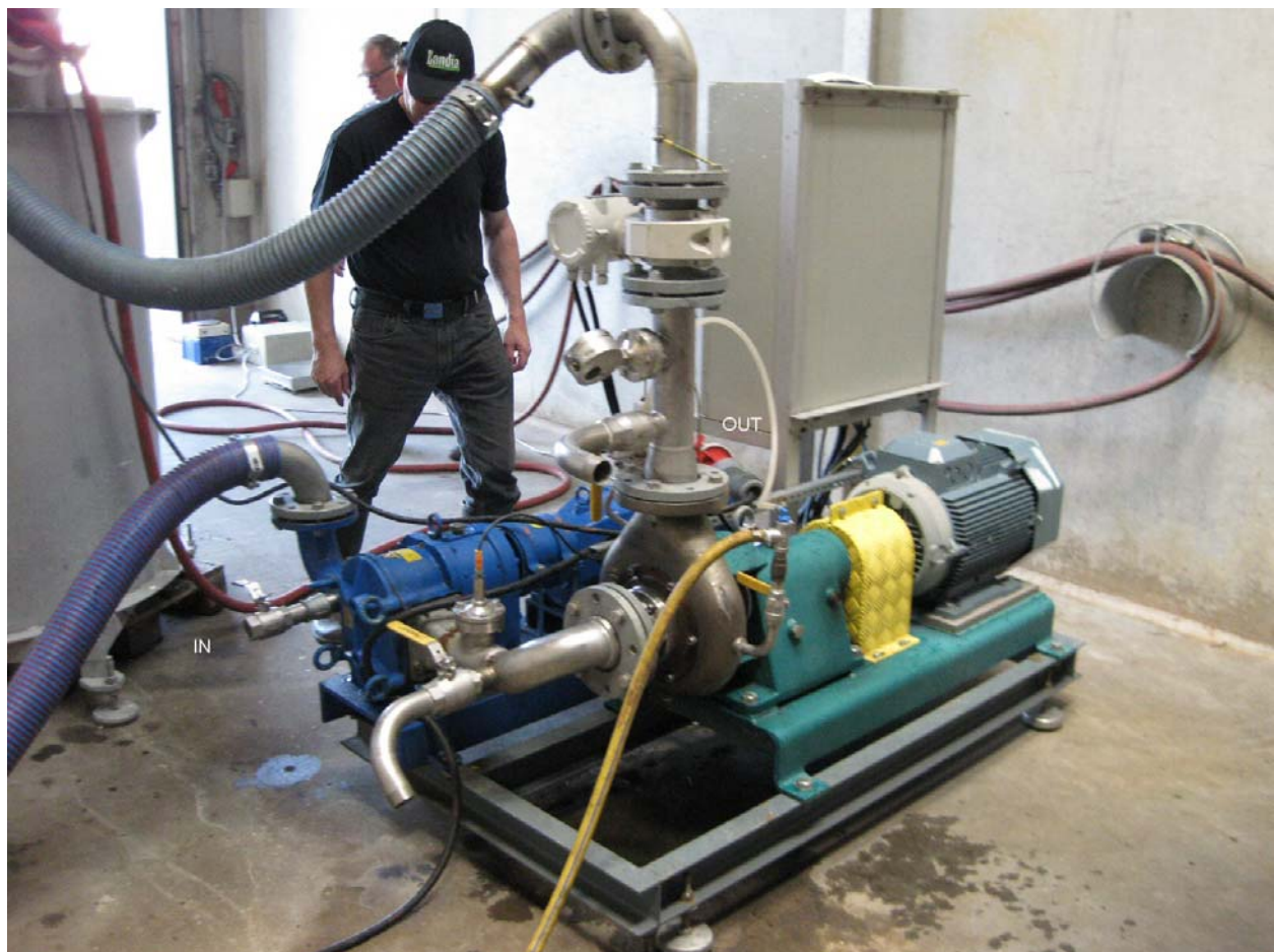
Figure 4 Deflaker GLD 200 Input sample valve in the middle
