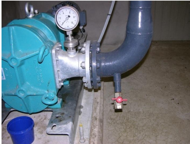
Figure 4. Tap for taking samples of input digested biomass.
