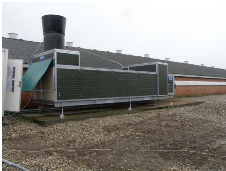
Figure 1. Picture of the Agro Clima Unit situated outside a poultry house. Ventilation air to and from the poultry house are drawn through the Agro Clima Unit by a countercurrent principle to utilise the heat content of out flowing air to heat up inflowing air.
