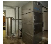
Iron generator and MDA
