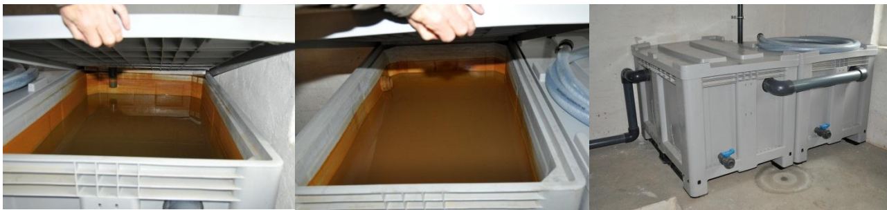
Figure 2-2 Pictures take during the site visit 26 th October 2011: from left to right 1) first desludging tank with backwash water inlet through the top of the tank 2) second desludging tank with outlet for decantate discharge to sewerage 3) desludging tanks with connecting pipe and bottom taps for sludge discharge; tank to the right with inlet pipe through the top of the tank and tank to the left with big outlet pipe to sewerage
