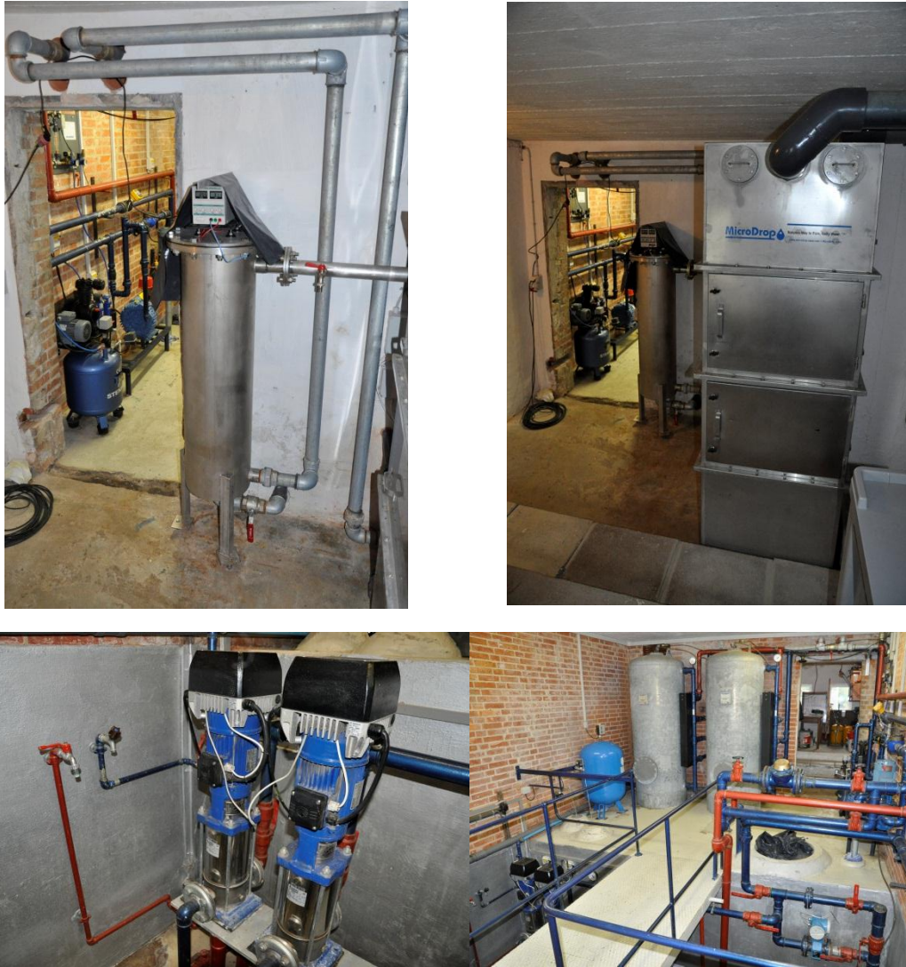
Figure 2-1 Pictures take during the site visit 26 th October 2011: Top left - of iron generator; top right - iron generator and aerator; bottom left – groundwater pumps and red/orange tap for groundwater and blue tap for drinking water; bottom right – inside the waterworks
