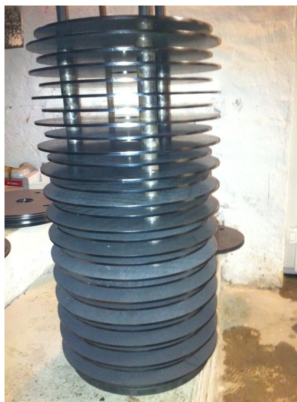
Figure 3-2 Pictures from the Utterslev-Kastager water works: 1) picture to the left: Iron generator in the background and aerator in the foreground 2) top right picture: two sand filters 3) bottom right picture: iron anodes and centre cathode before installation in the iron generator
