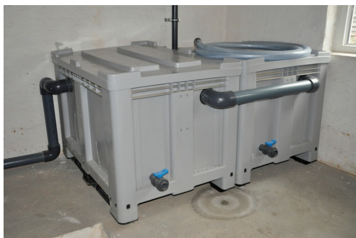
Figure 3-3 Desludging tanks at the Utterslev-Kastager water works
