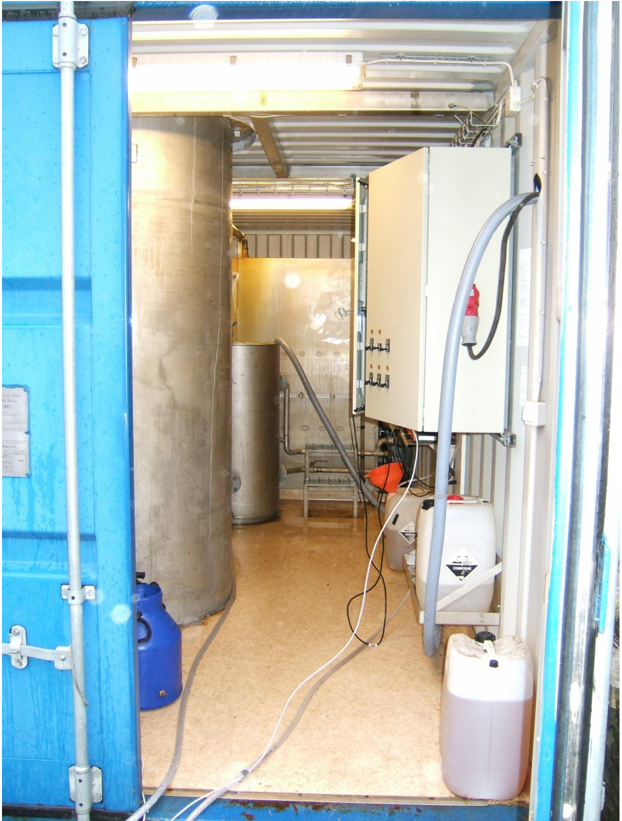
Figure 2-3 View into the container. On the left hand side is the cylindrical multi-media up-flow filter, in the back the large rectangular tank for backwash water.
