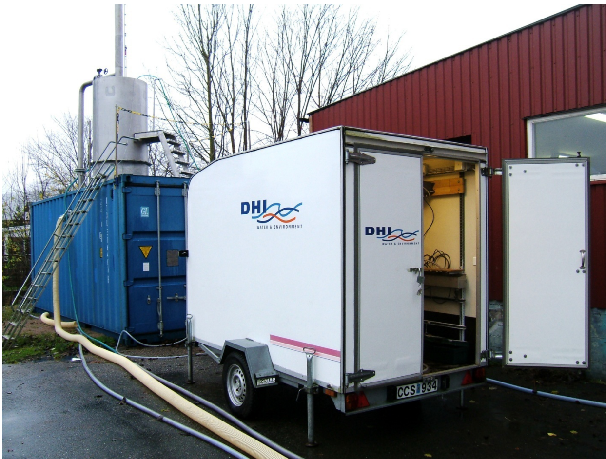
Figure 2-2 Rosfilter pilot plant and DHI's trailer with analytical equipment at Lilla Edet water works.
