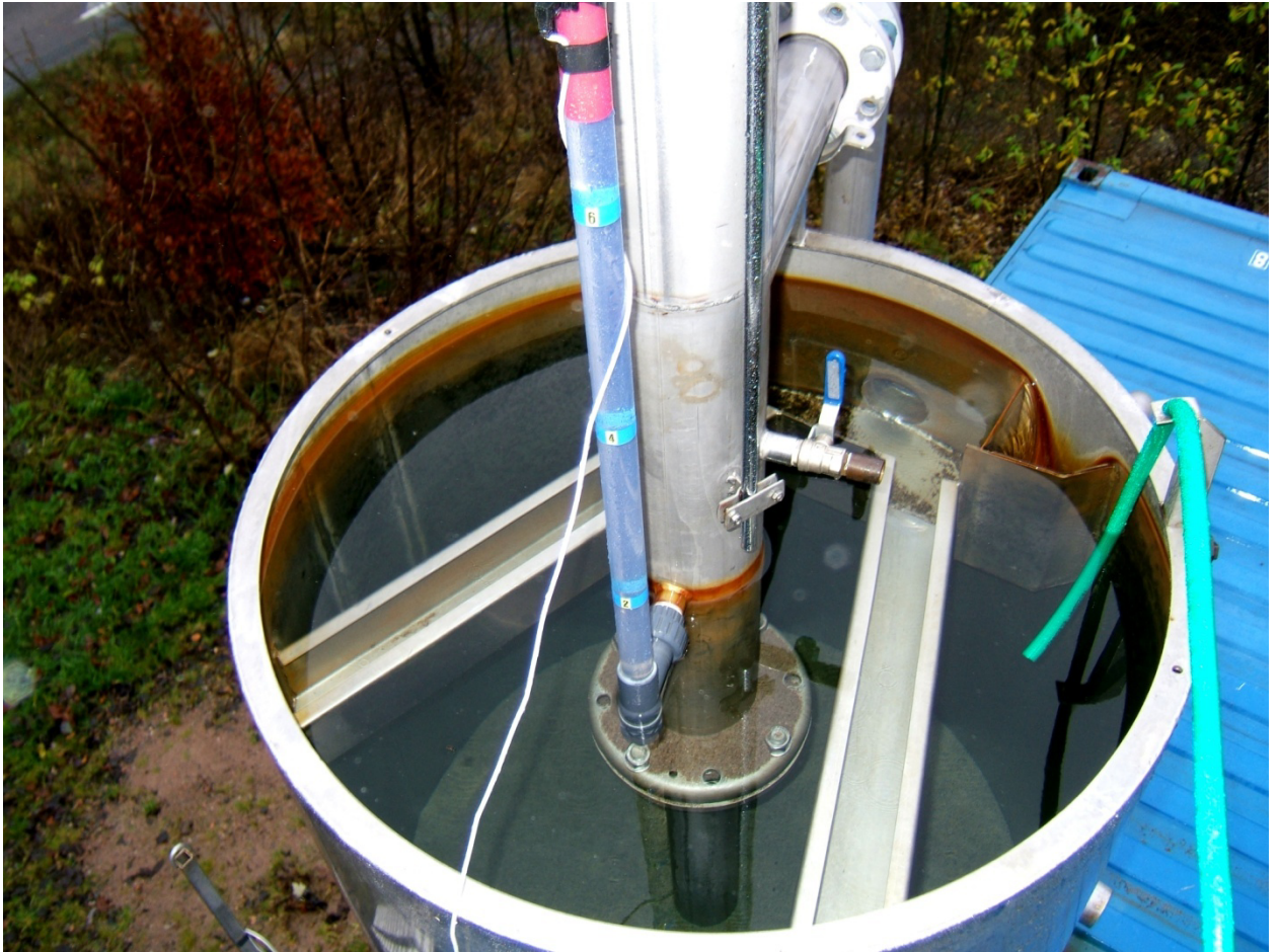
Figure 2-4 View of the filter protruding from the top of the container. The transparent pipe contains the switch that triggers the backwash at a pre-set headloss.
