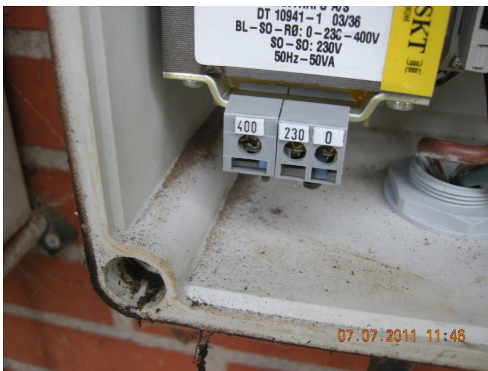
Dust inside slurry pump control cabinet
