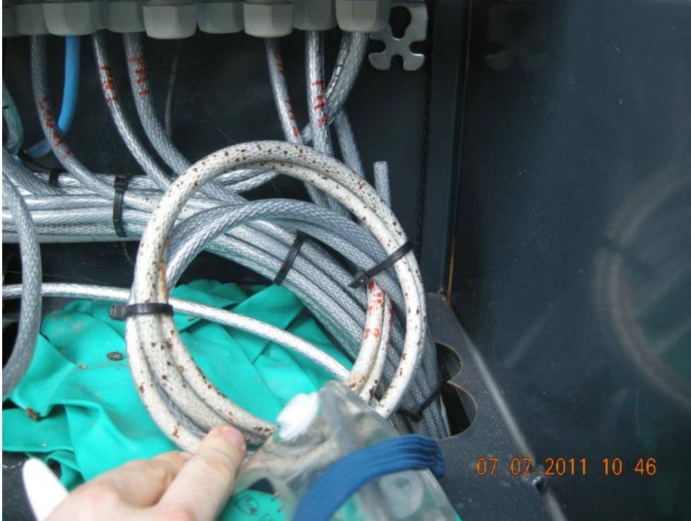
Electrical wires in bottom of control cabinet in contact with sharp edge in the bottom plate
