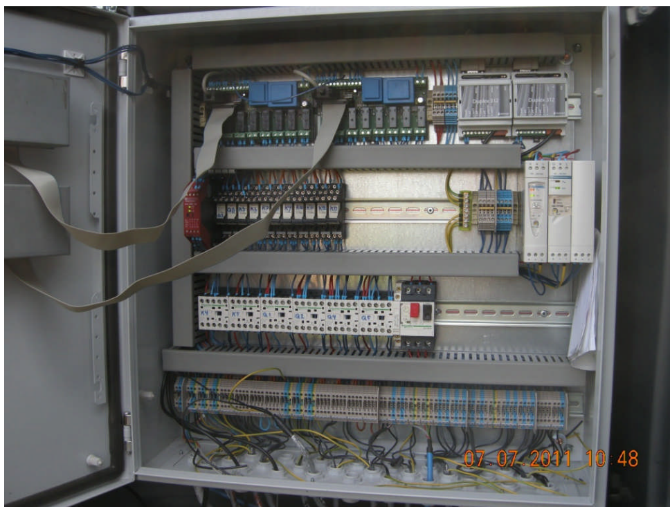
Inside cabinet for electronics
