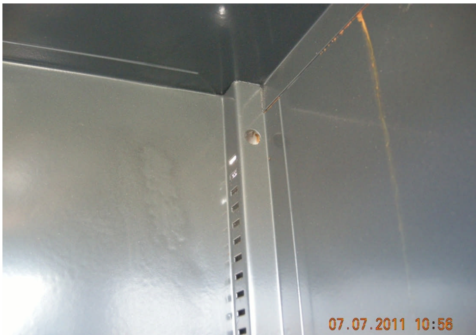
Corrosion near top of control cabinet
