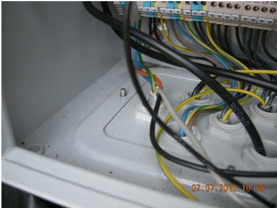
Cable entry into cabinet for electronics
