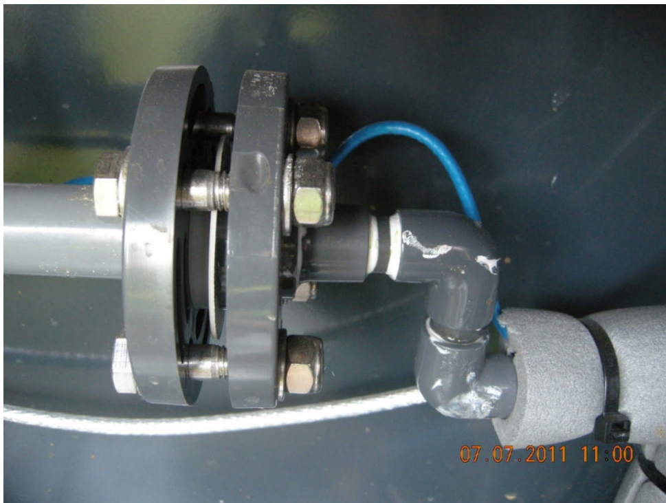
Blue heat trace cable not in good contact with tubing and flanges
