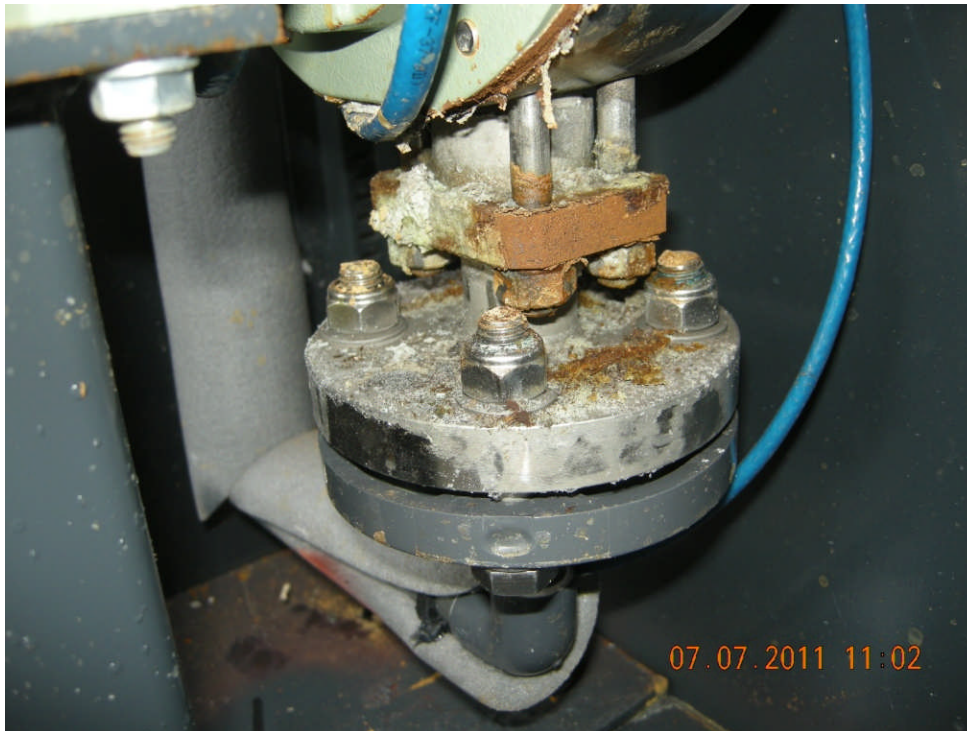
Corrosion attack below pump unit
