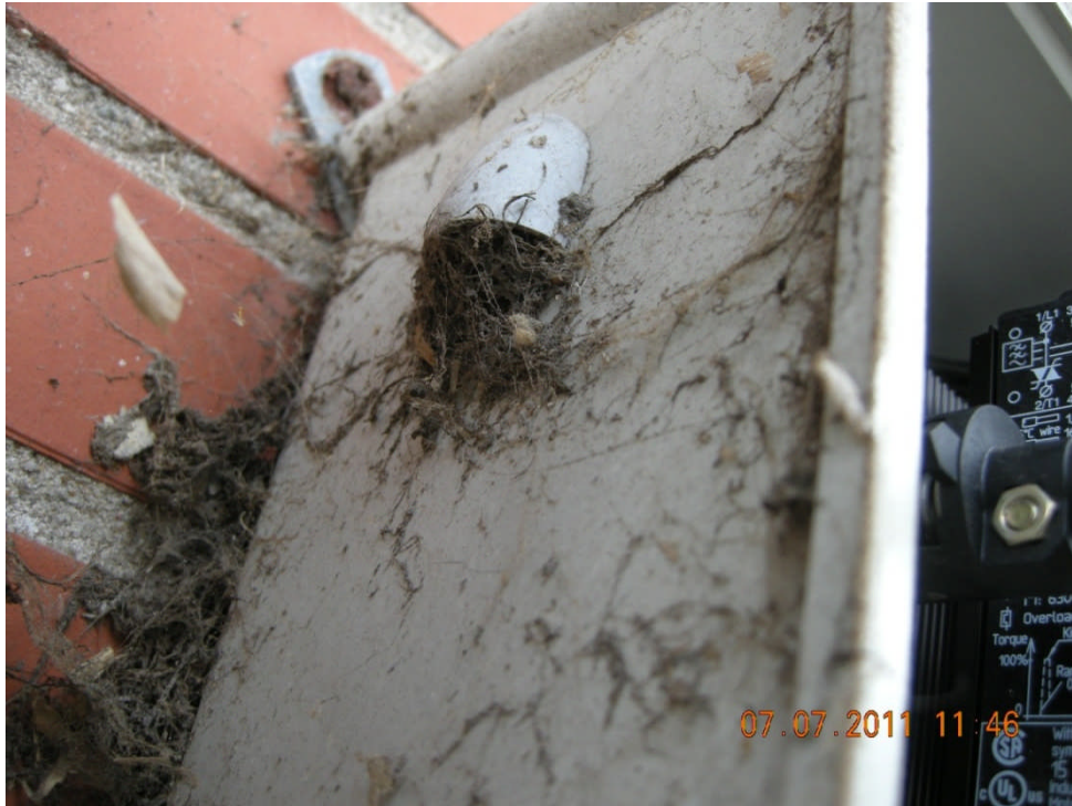
Ventilation opening on the side of the old slurry pump control box
