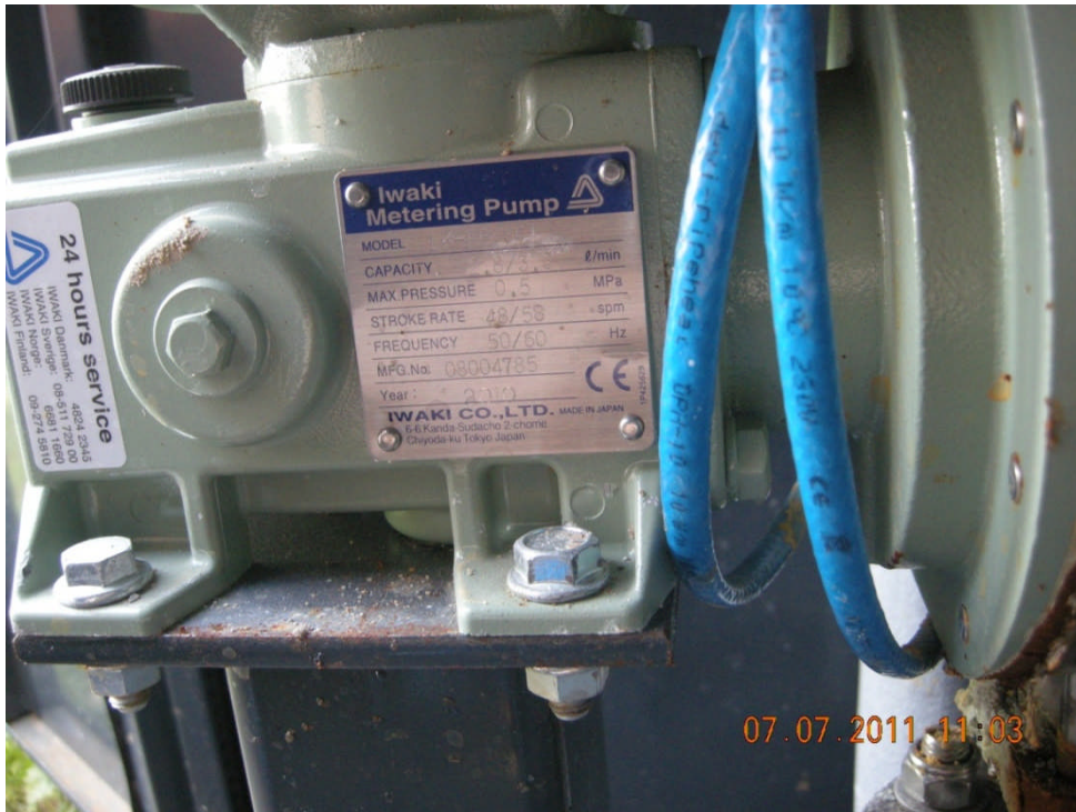
Blue heat trace cable not in good contact with pump housing
