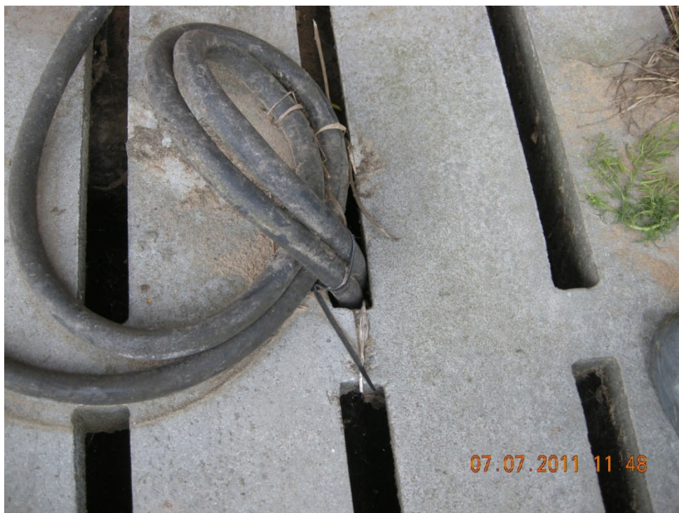
Supply wires for pumps in slurry tank close to sharp edges in the concrete plate
