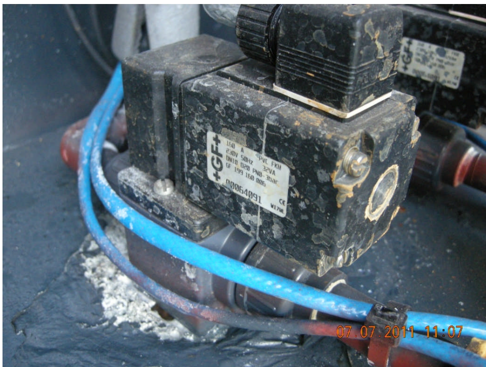
Corrosion attack on and below valve
