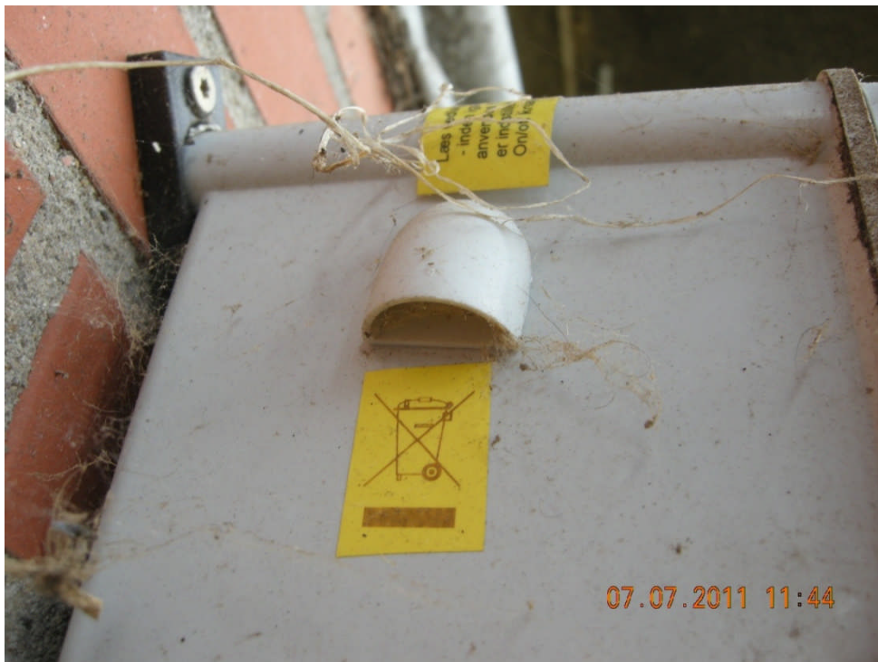
Ventilation opening on the side of the new slurry pump control box
