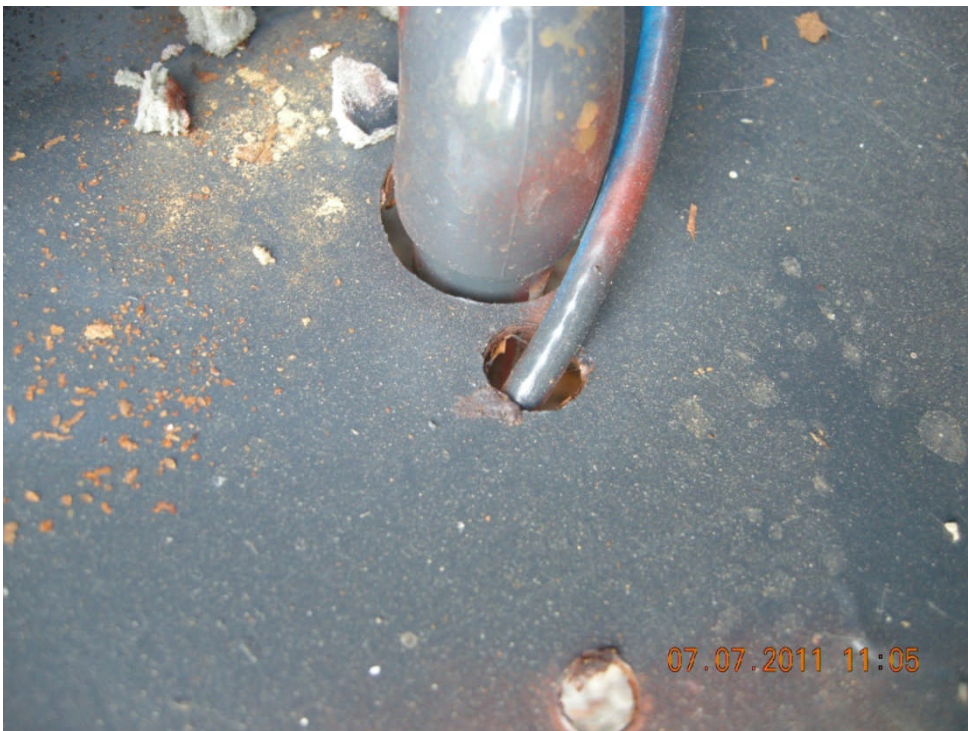
Heat trace cable in bottom of control cabinet in contact with sharp edge in the bottom plate
