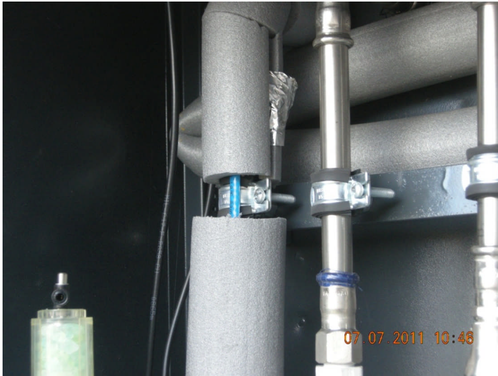
Blue heat trace cable inside thermal insulation: Good
