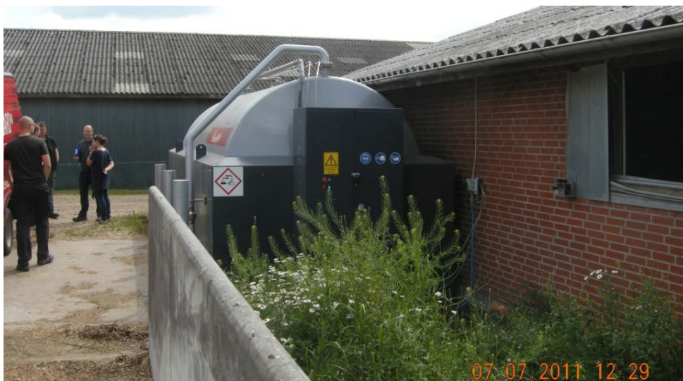
Acid tank and control cabinet
