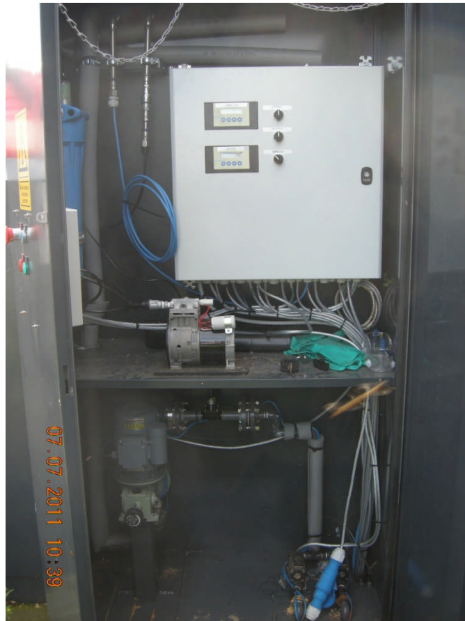
Inside control cabinet
