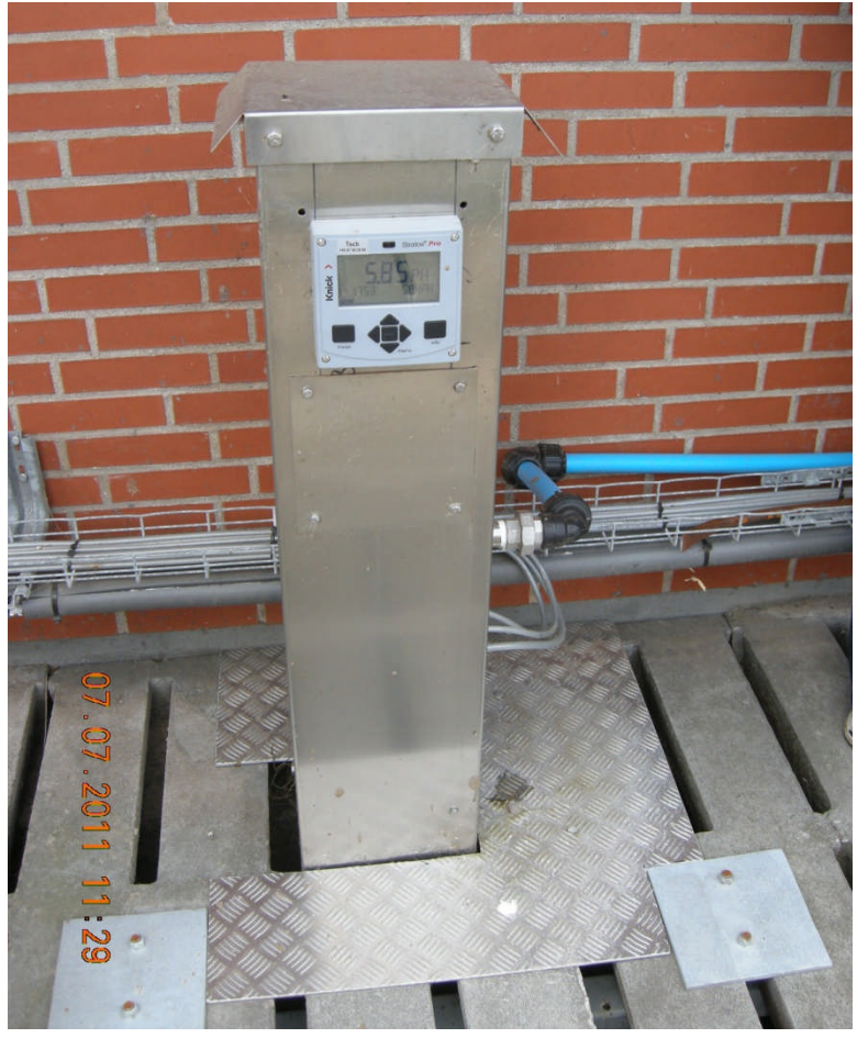
Cabinet with pH electronics on top of slurry tank
