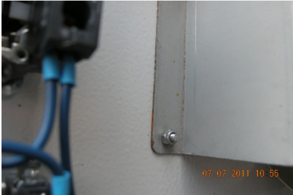
Corrosion on edge of mounting bracket
