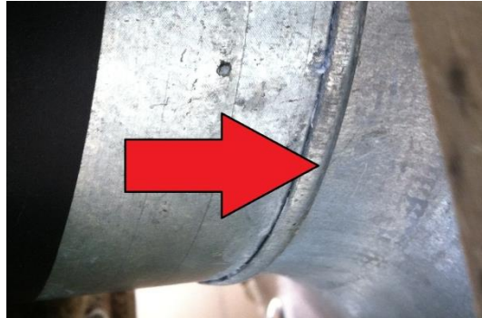
Figure 1 - Snug fit in the transition between air heater outlet and measuring pipe
